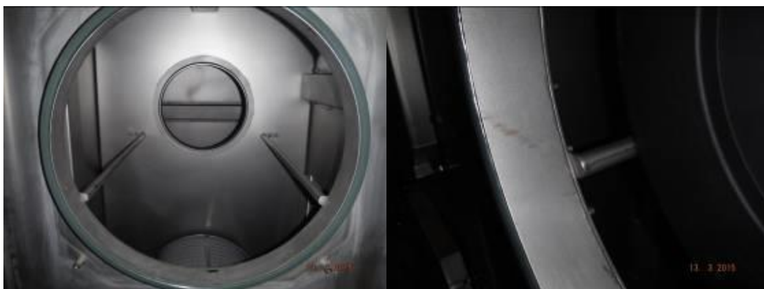
Fig 11. Guide Rails With Insufficient Corner Rounding.
