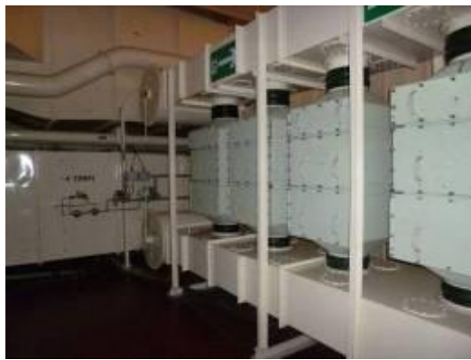
Fig 3. Shows the “walk in” style of filter plant room, where the filter is simply withdrawn into the room with no protection as the whole room was classified as a dirty area.
