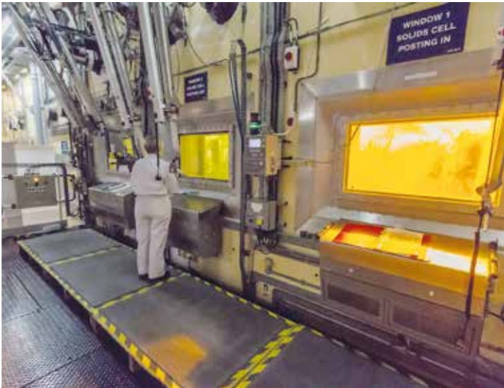
Figure 4 - An operator processes historic raffinates from the fast reactor fuel reprocessing cycle. The cells are used to mix raffinates with cement powder to create a quality waste product that is passively safe
