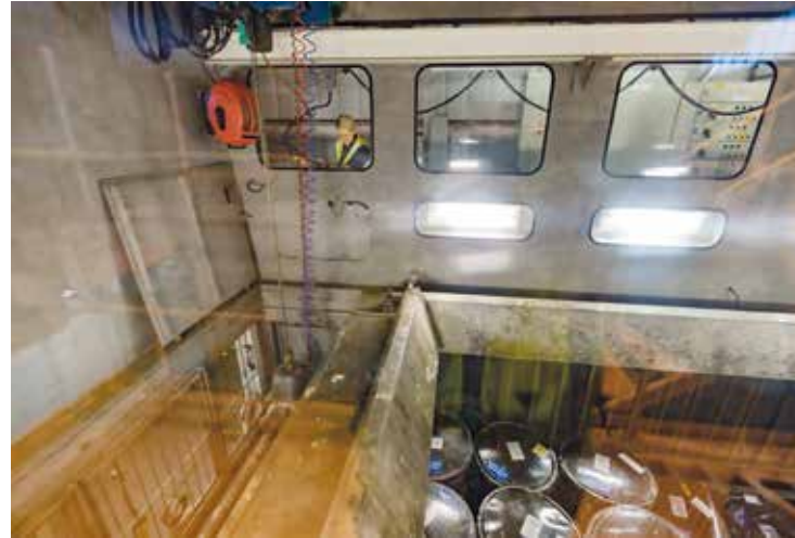
Figure 3 - Inside the Waste Receipt, Assay, Characterisation and Supercompaction facility (WRACS), an operator loads pucks (compacted C-Bins containing LLW) using a remotely controlled grab into a half height ISO container, destined for grouting prior to disposal in the vaults. Supercompaction of the C-Bins allows for more C-Bins per container and is an example of one of the many ways Dounreay optimises its waste management operations
