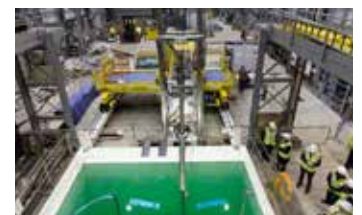
EPC for Fuel Handling and Fuel Inspection Systems – Ignalina NPP, Lithuania
